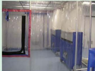
Figure 3: AHU (-ve Pressure)
