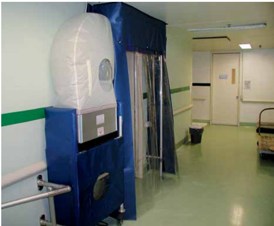
< LOW PROFILE POSITIVE PRESSURE ANTEROOM USED AS AIR BARRIER IN HIGH TRAFFIC CORRIDOR
