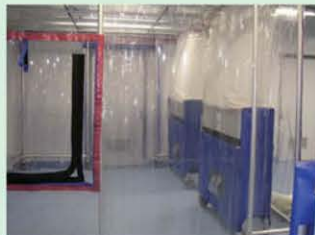
Figure 3: AHU (-ve Pressure)
