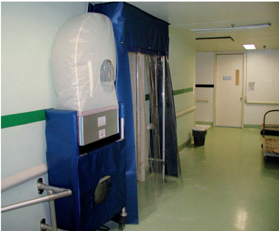
< LOW PROFILE POSITIVE PRESSURE ANTEROOM USED AS AIR BARRIER IN HIGH TRAFFIC CORRIDOR
